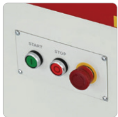
Main Control Panel with Emergency Stop
