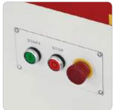
Main Control Panel with Emergency Stop
